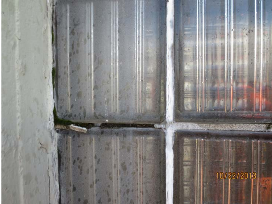
Photo No.7 Missing sealant around glass blocks
