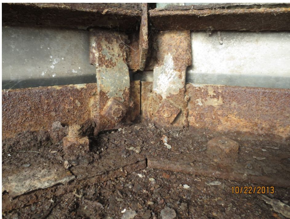
Photo No.4 Corrosion of steel framing members
