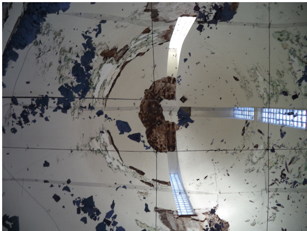
Photo No.9 (Looking Up) flaking paint and missing sections of stucco material
