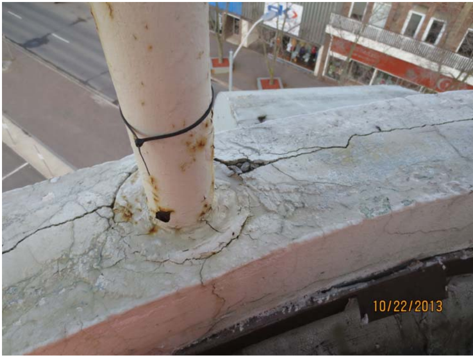
Photo No.2 Deteriorated/delaminated concrete parapet wall & metal railing
