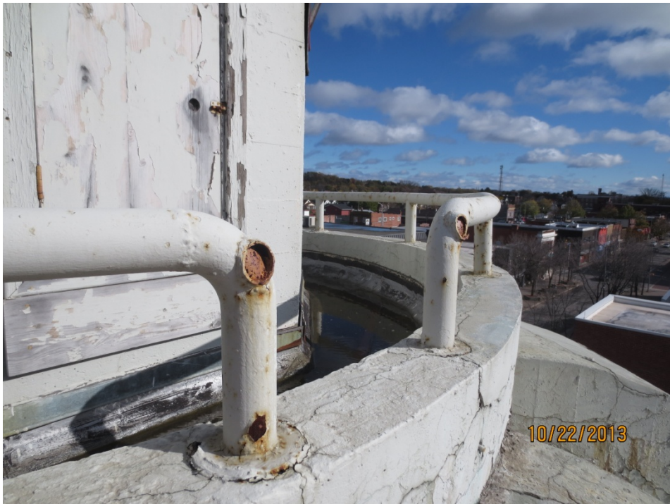
Photo No.1 Deteriorated concrete parapet wall and horizontal surface of buttress
