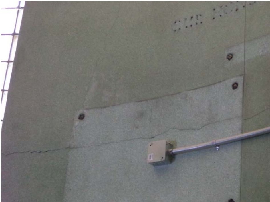
Photo No.8 Full perimeter crack in Terrazzo wall finish
