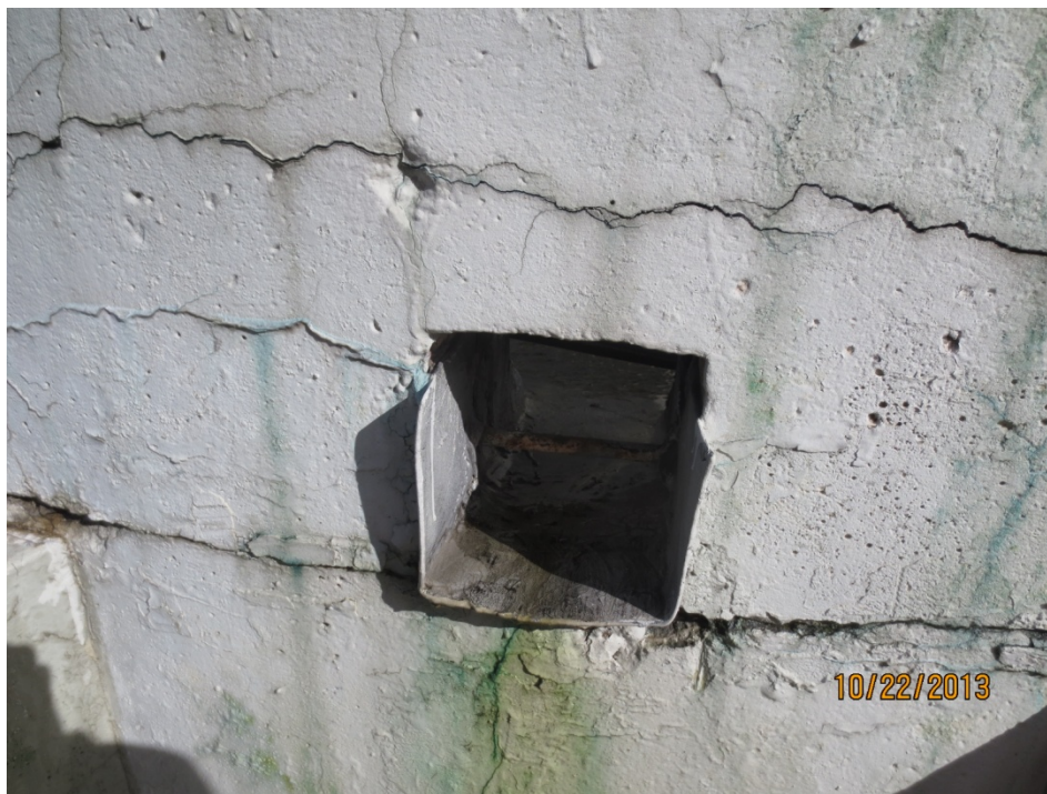
Photo No.3 Deteriorated/delaminated concrete parapet wall and drainage scupper
